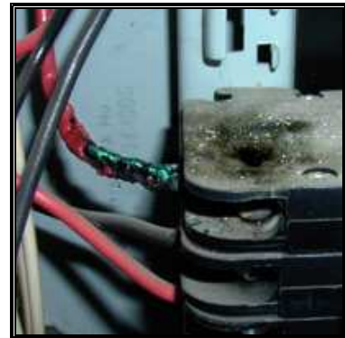
Stab-Lok breaker casing (blow out)
