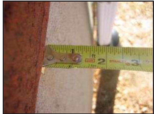
3.0 Picture 2 - Top SW corner of rear wall.
